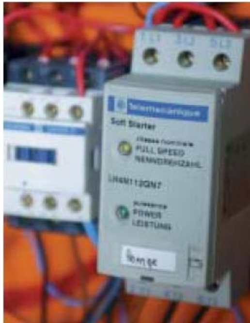
Figure 3. Electronic "Soft" Starter for Electric Motors
