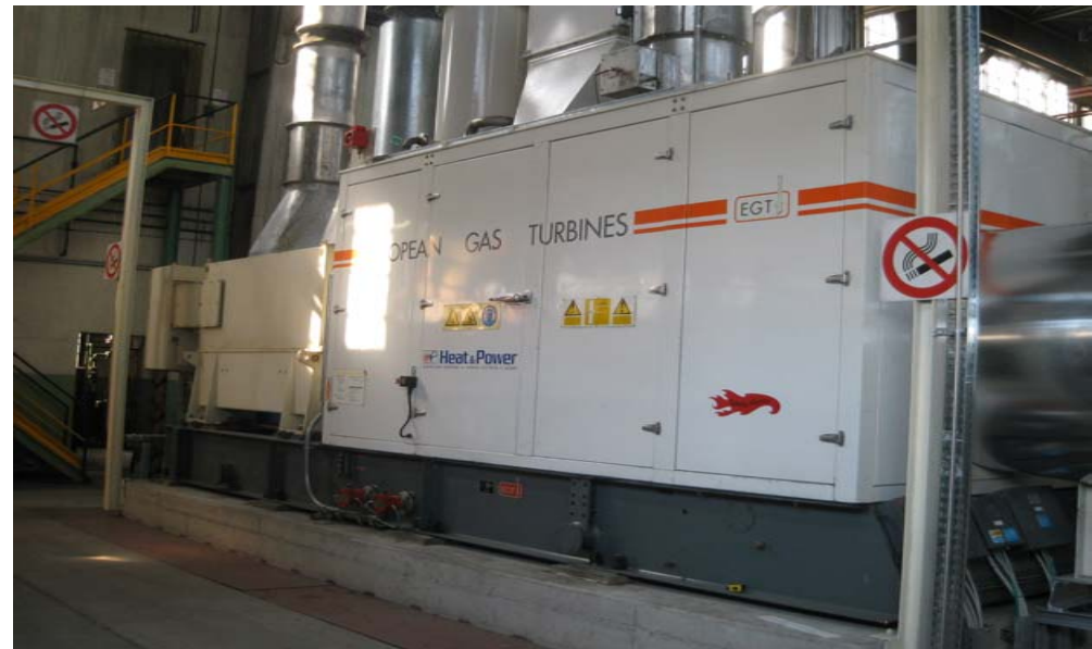
4.800 kW GT Cogeneration Plant
