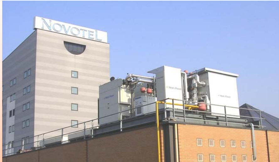
130 kW mGT trigeneration Plant
