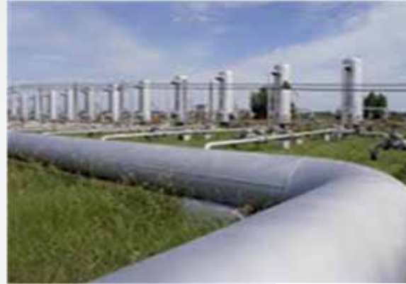
Fig.3 Natural gas supply
