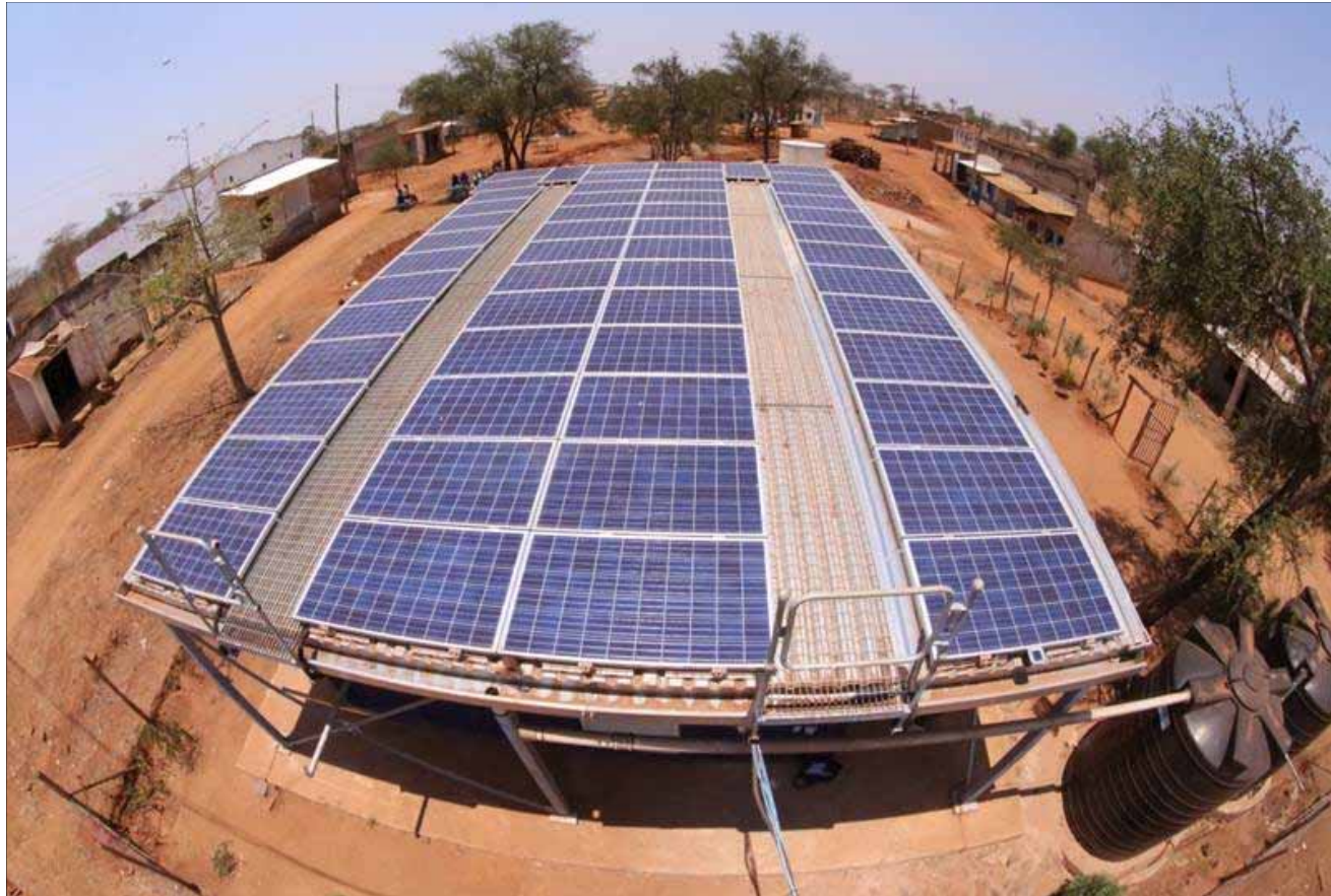
Bird's eye view of the 13.5 kW PV system in Makueni County, Kenya.
