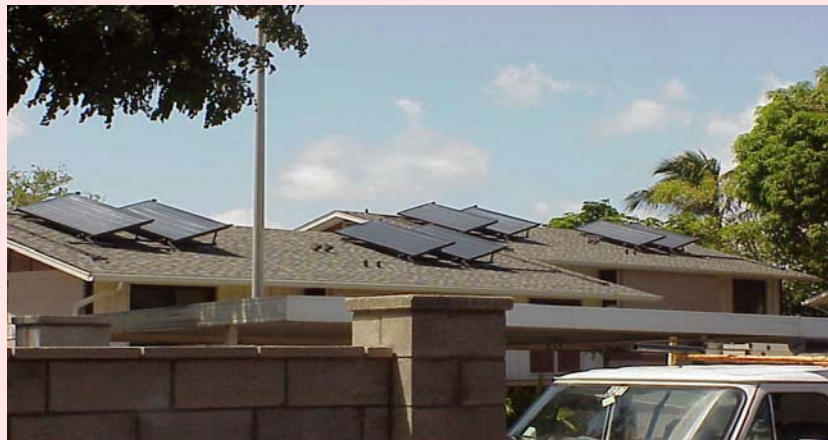
Figure 42: Solar water heating systems on USCG housing in Hawaii.
